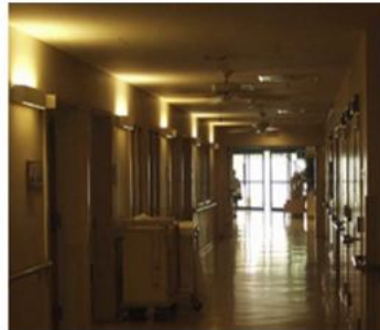
Figure 1: An example of lighting problems a) glare from doors at the end of the corridor, b) uneven lighting, and c) low light levels.
